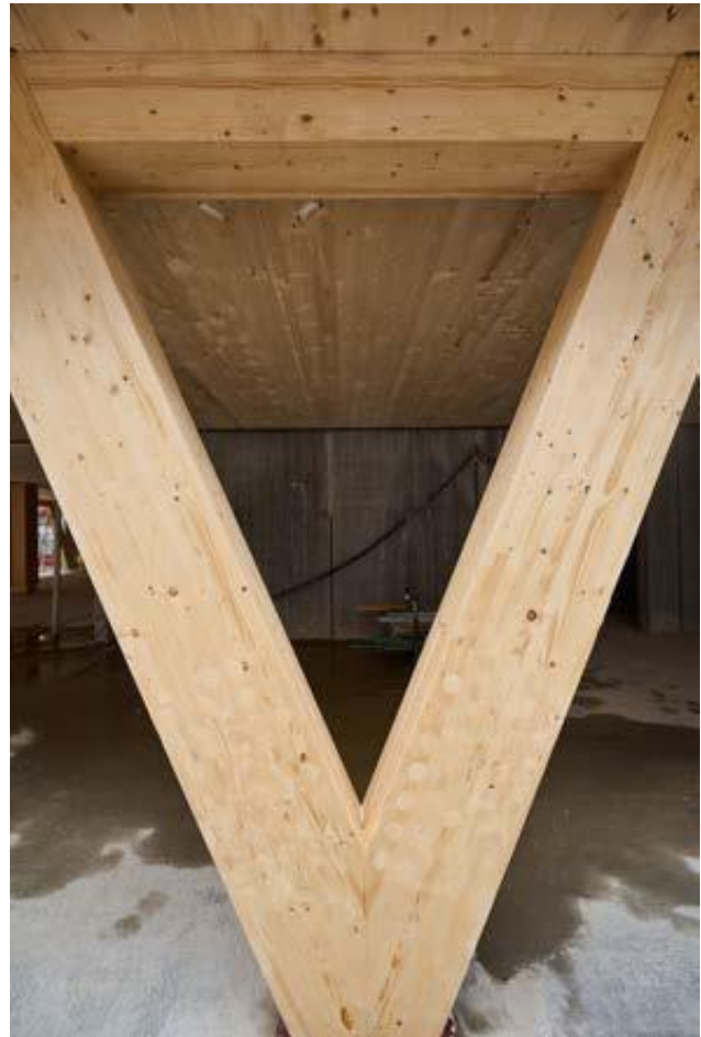
► Detail of the innovative timber structure of the office building Montoyer 10 - Brussels' CBD (BE)
